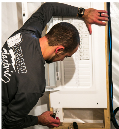
Corey Prehoda installing the clear cover door on the Leviton Load Center
